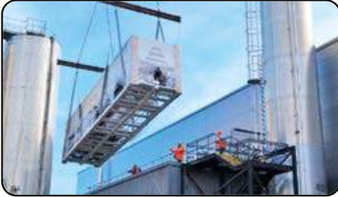
* Chiller installed in UK, 1070 kW
