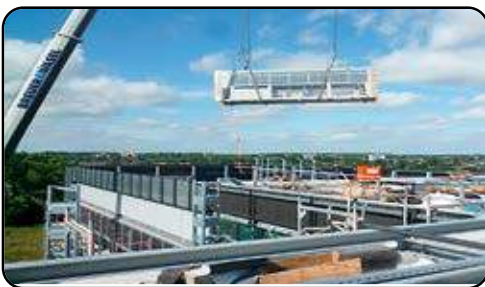
* Chiller installed in Dusseldorf, Germany, 820 kW
