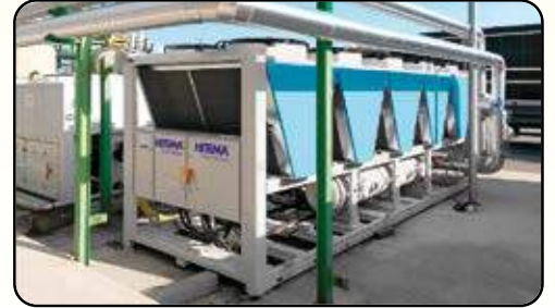
Chiller with Turbocor compressors, installed in Spain, 780 kW
